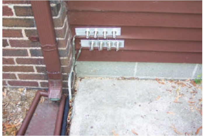
Outside View Of Bulkhead Connectors
